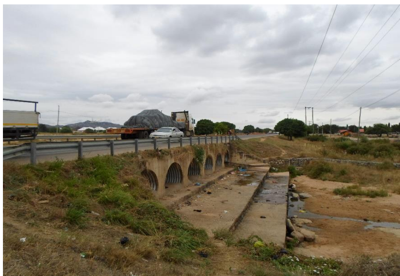
Fig. 17 Ilazo-Ipagala Storm Water Drain
