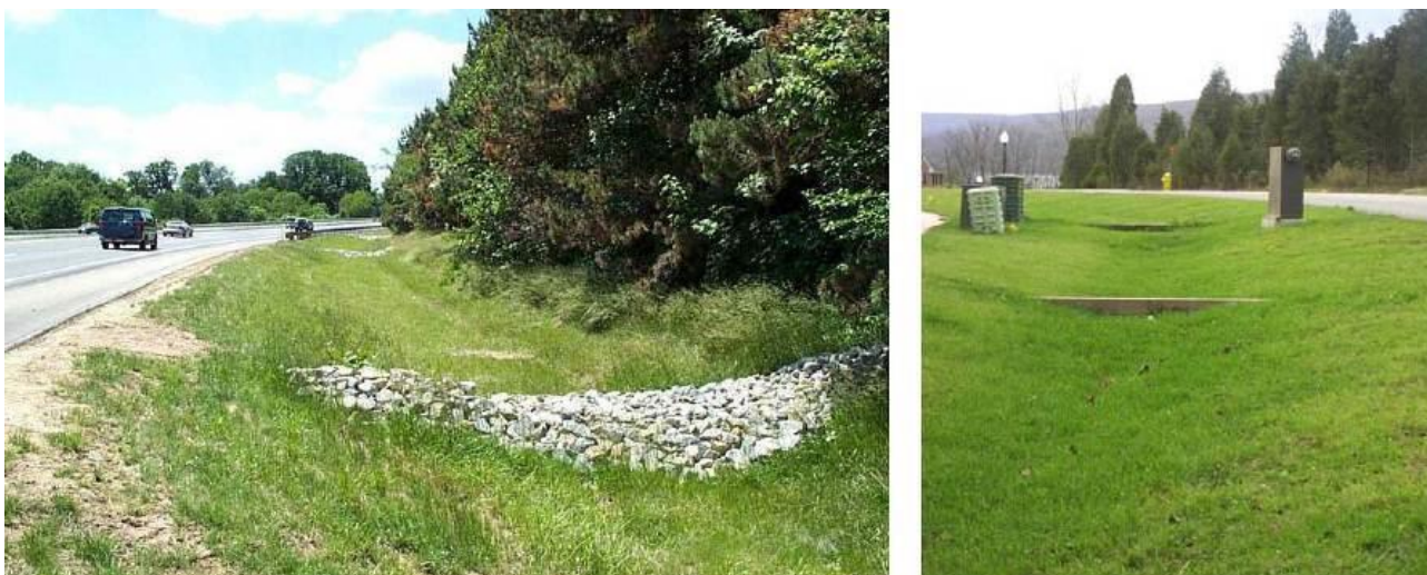
Fig. 41 Check Dams along the Main Storms
