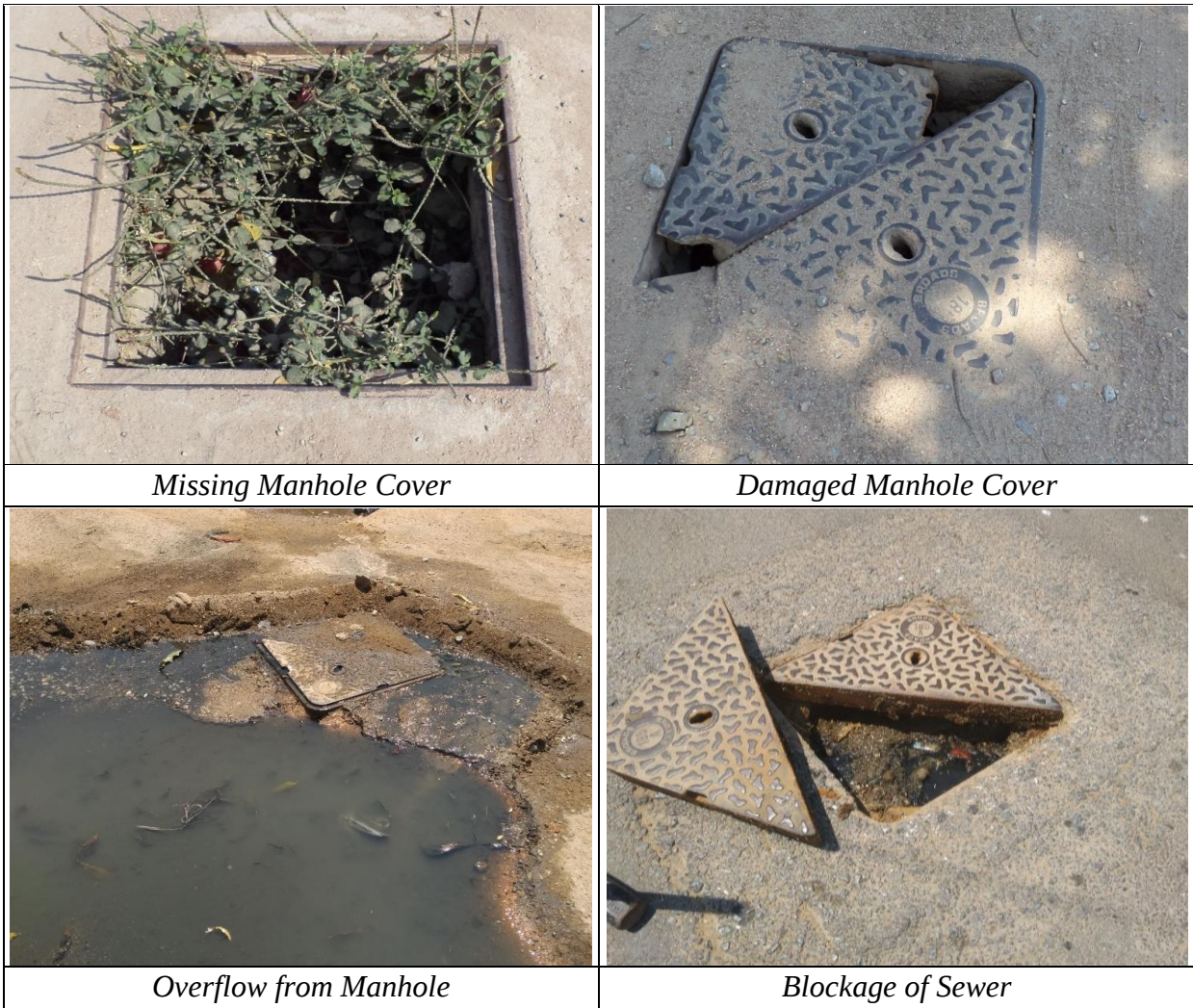
Fig. 114 Problems on Sewer and Manholes
