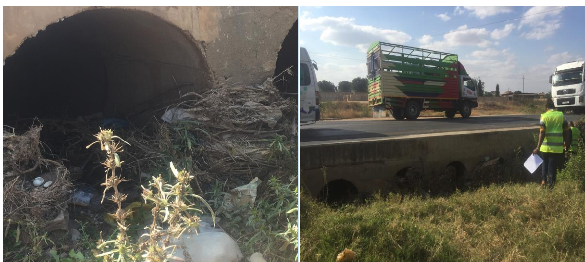
Fig. 35 Culverts blocked with Debris Materials
