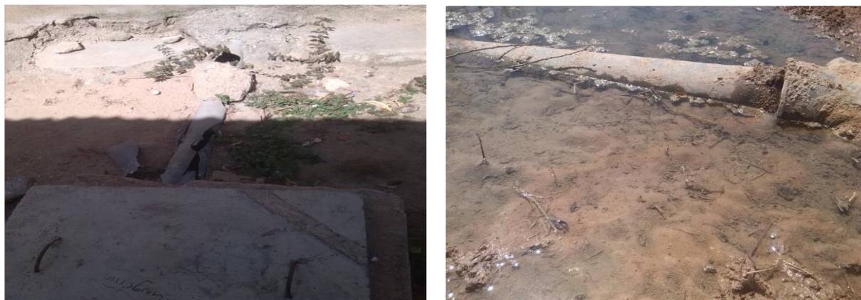
Fig. 1 Exhausted Sewerage System in Dodoma city
