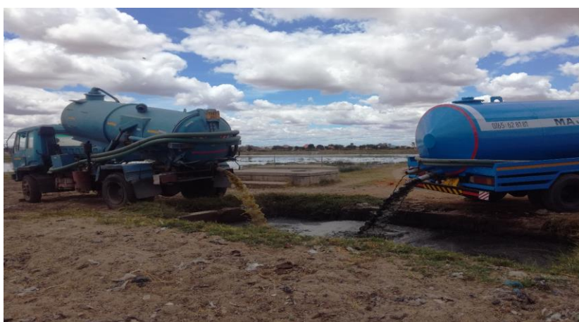
Fig. 117 Vacuum tankers discharging Fecal sludge at the disposal point
